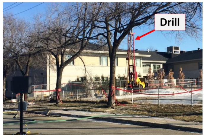
Figure 1 Visible image of the shale gas leak site as seen from the sensor location.
